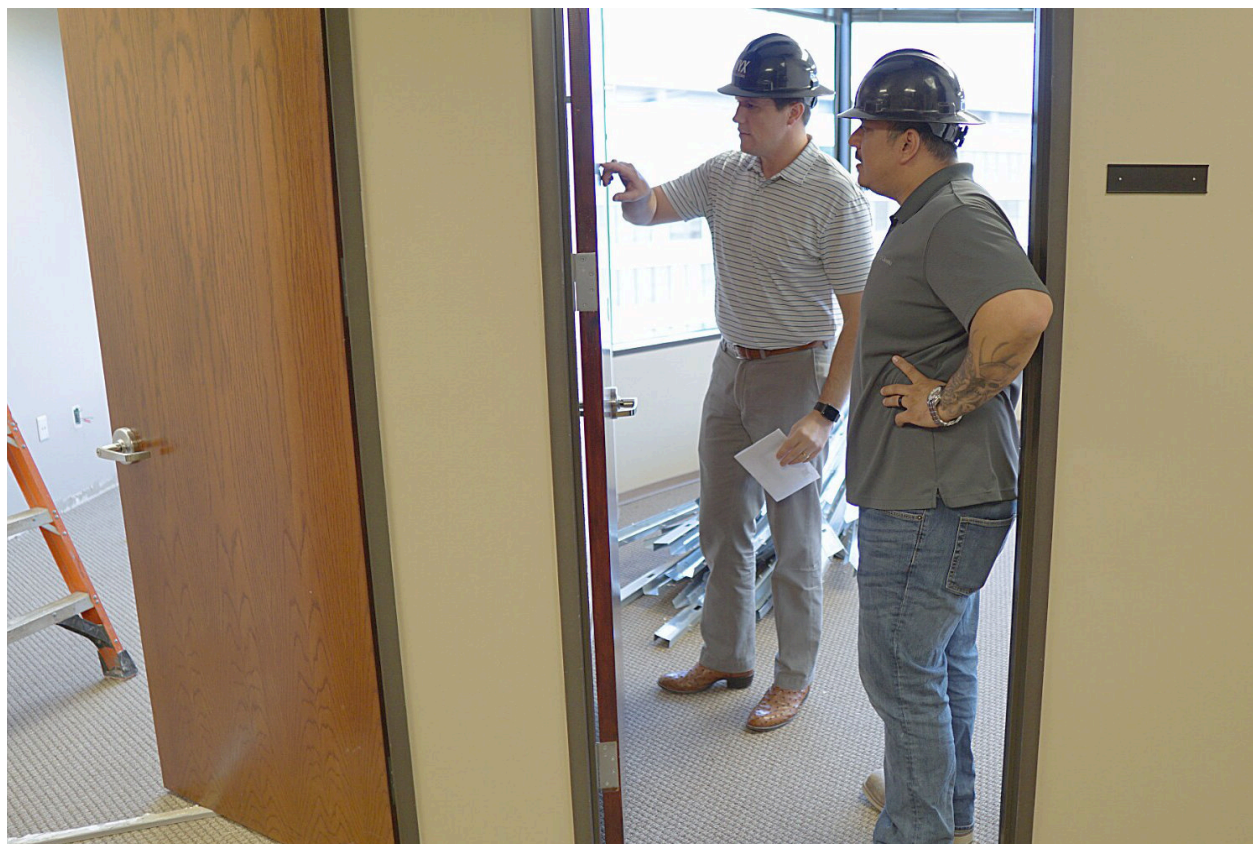
Materials, labor, and oversight are coordinated to ensure timely completion of each task.
